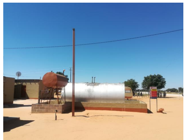
Photo 4. Existing aboveground diesel tank
