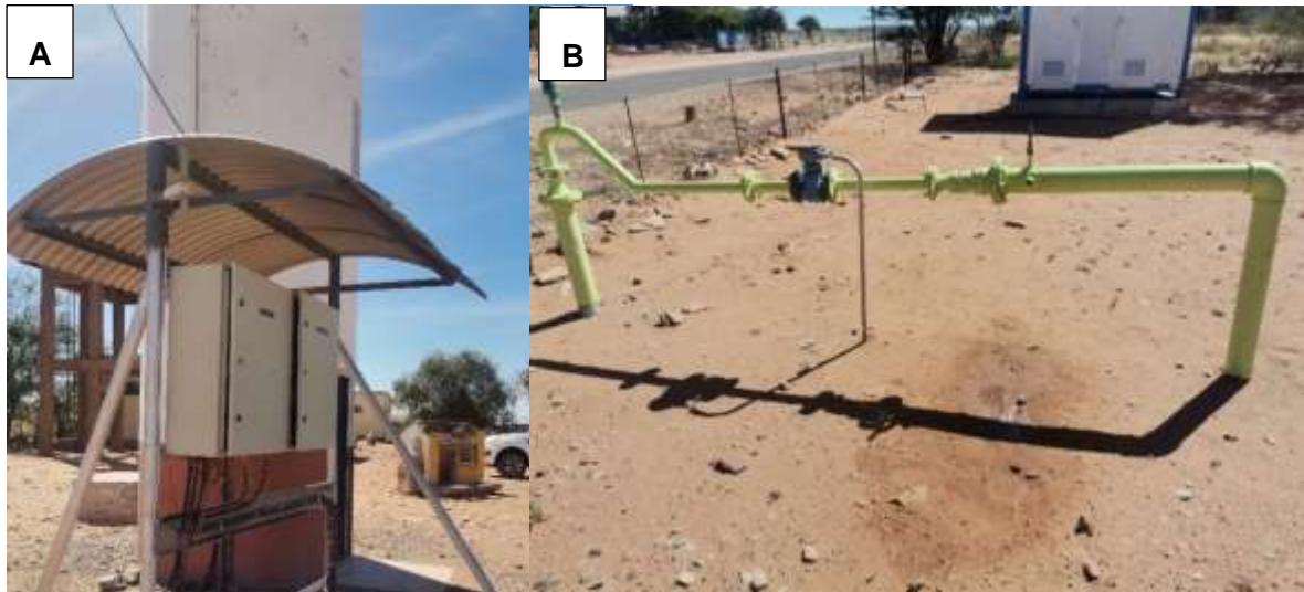
Figure 9: Elevated Tower and control system
