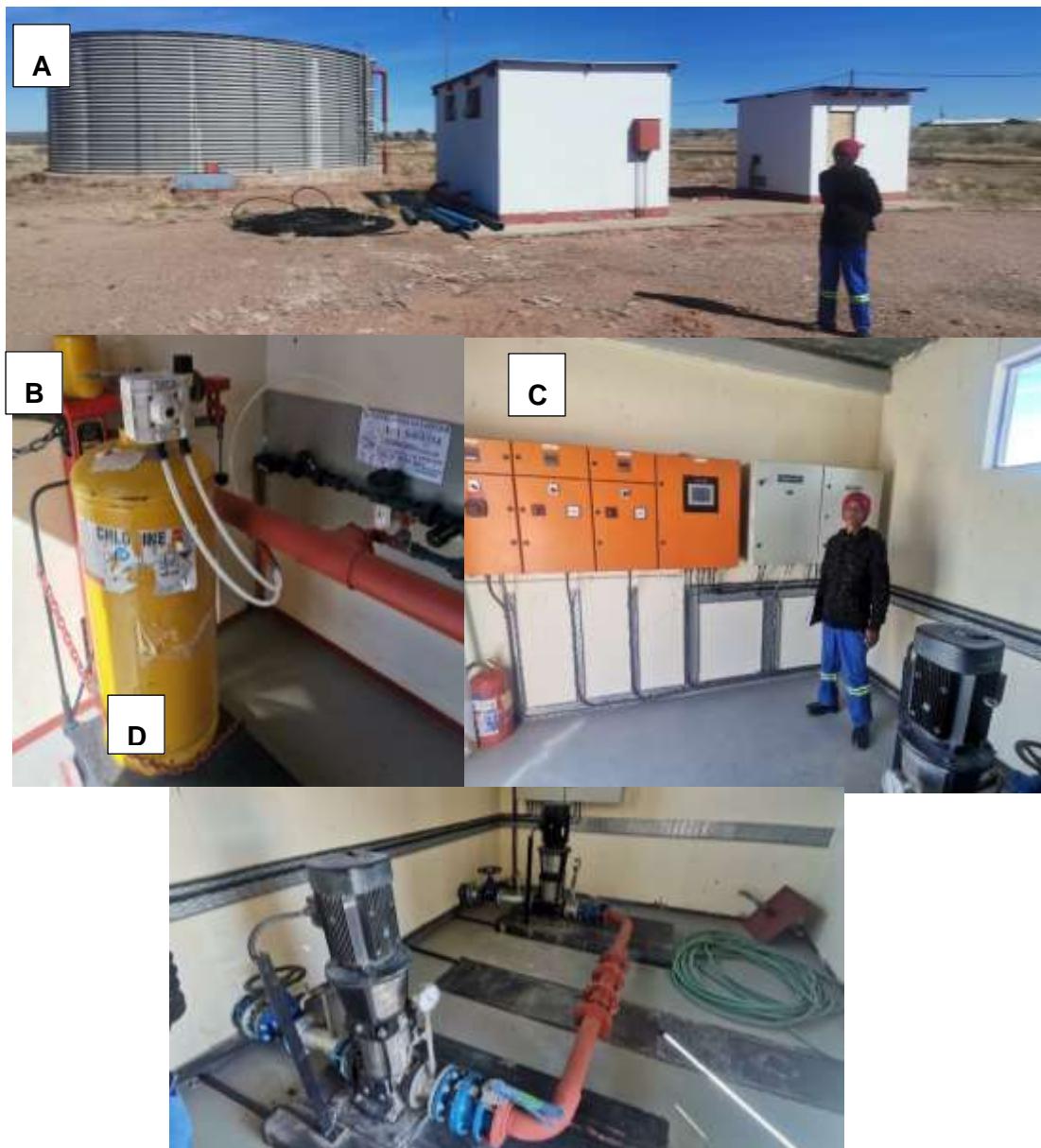
Figure 8: Bulk storage infrastructure
