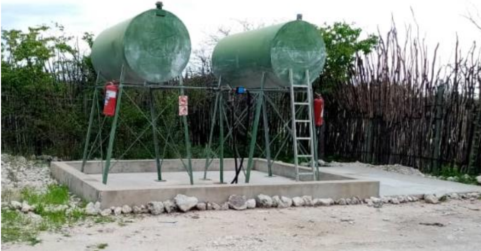
Figure 7. Diesel tanks mounted on a bunded cement floor.
