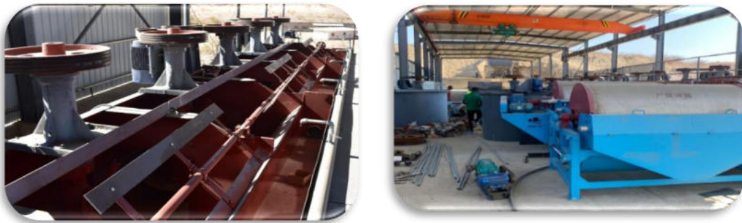
Figure 3:3 Sections of the copper floatation process structures in the plant
