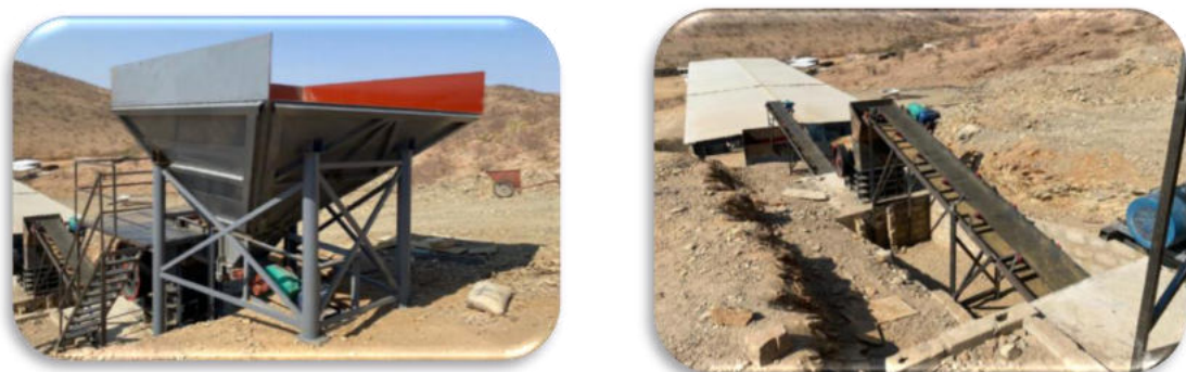
Figure 3:2 Constructed sections of the low-grade ore processing plant by floatation
