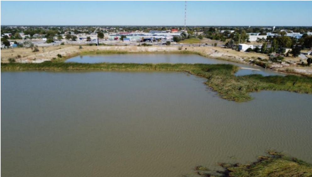
Figure 4-4 Aerial photograph showing different levels of freeboard in the main section and the side-section
