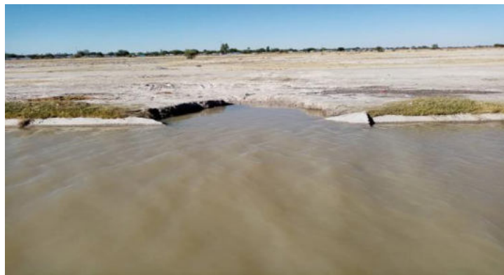
Figure 5-4 Damage along the canal near Oshakati
