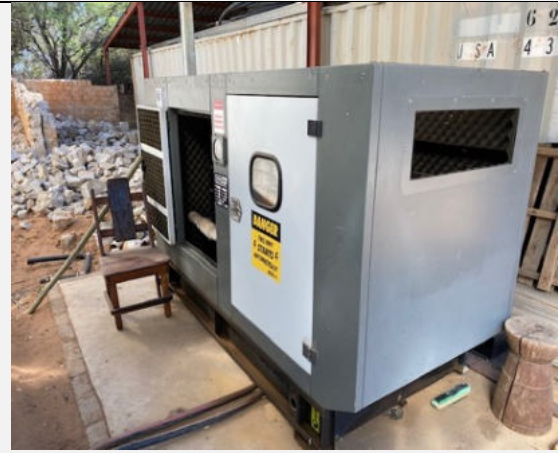
2 x 100 kW backup diesel generator.
