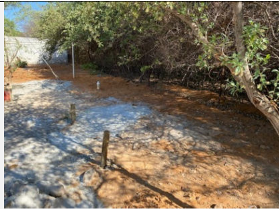
Soak away, part of the sewage system.
