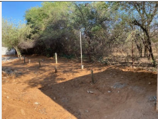
Soak away, part of the grey water system.
