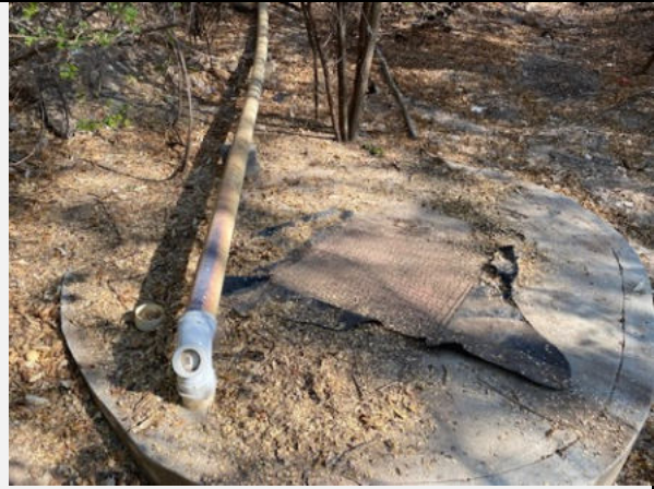
Holding tank for a greywater system.
