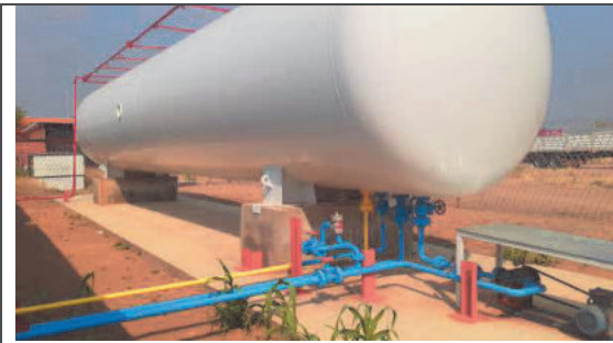
Photo 2-1 LPG Storage tanks with fire protection
