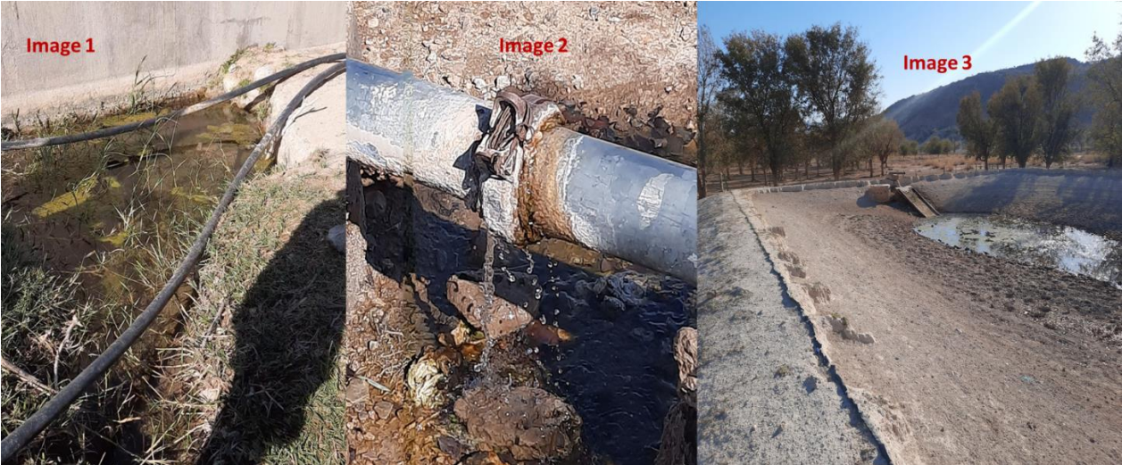
Figure 1: Image 1 - Silted water abstraction weir at the source, Image 2 - Water leakages along the pipeline, Image 3 - Heavily silted water storage earth dam at Warmquelle. The pond is poorly
