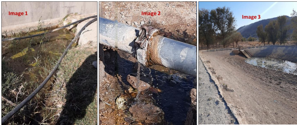
Figure 1: Image 1 - Silted water abstraction weir at the source, Image 2 - Water leakages along the pipeline, Image 3 - Heavily silted water storage earth dam at Warmquelle. Source: Own images taken during field visit.
