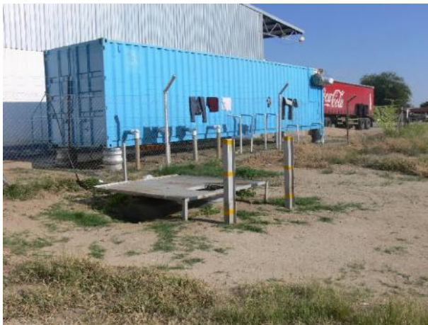
Photo. 3.3.7 Ablution and septic tank of Portion 18
