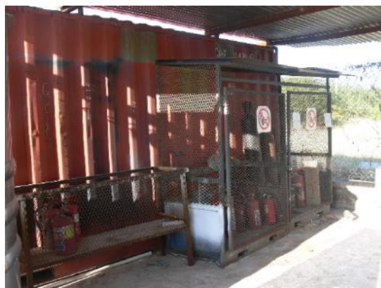
Photo 3.4.6 Fire extinguishers on site
