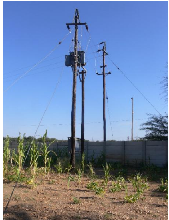
Photo. 3.3.2 Electricity connection to Portion 22
