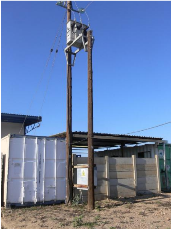
Photo. 3.3.1 Electricity connection to Portion 18
