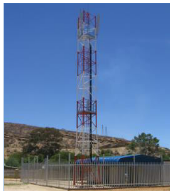
Figure 2: Example of the Lattice Tower ( https://powercom.na/ )
