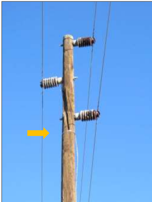
Figure 7-2: Example of "gapping" of a pole earth wire to provide an air space safety gap, in order to reduce the electrocution risk, The arrow indicates the upper limit of the earth wire.
