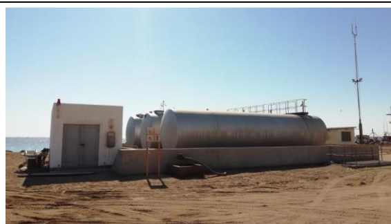
Photo 1. Illuminating paraffin storage tanks
