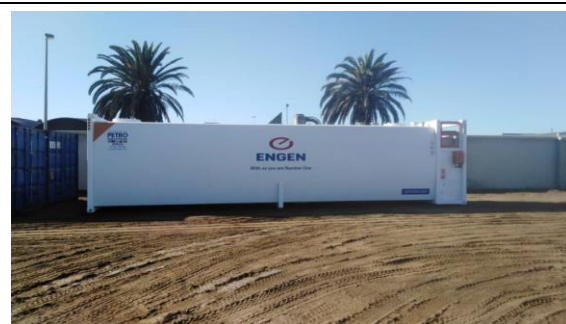
Photo 2. Example of self-contained diesel tank
