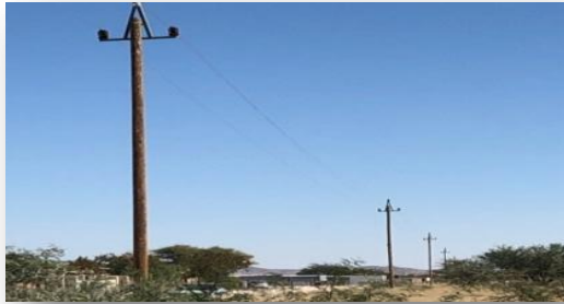
Figure 7: Electricity Poles and Streetlight on Portion 5
