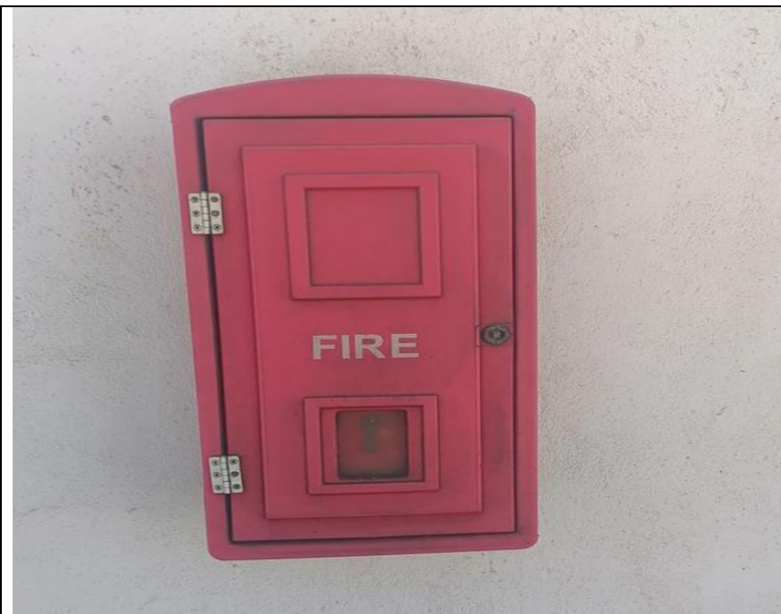
Fire Hydrant at site
