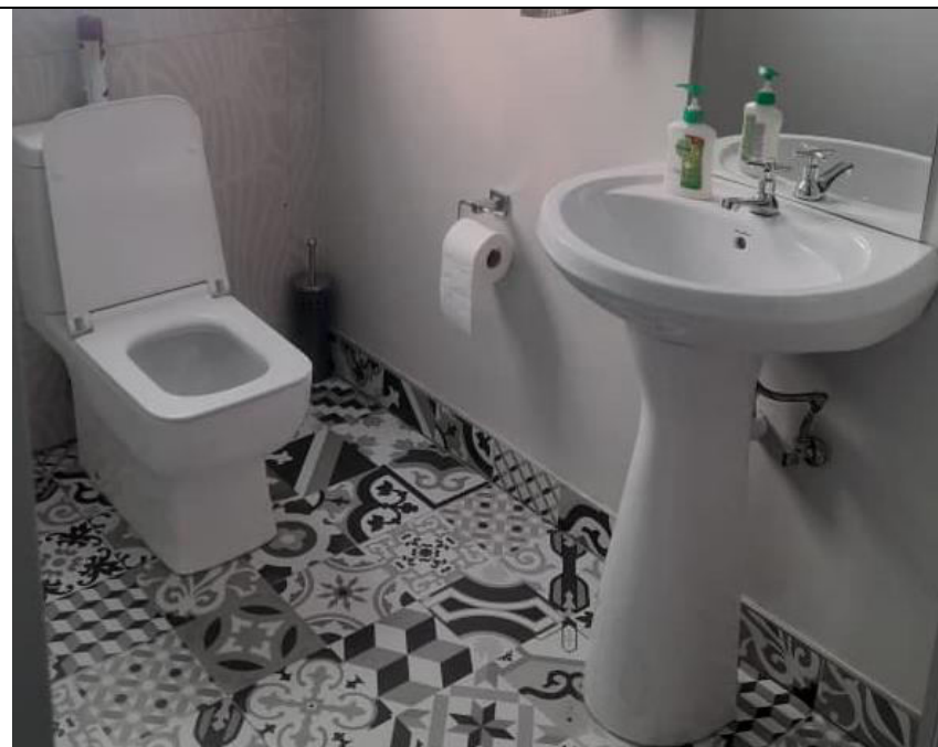
Staff Ablution facility
