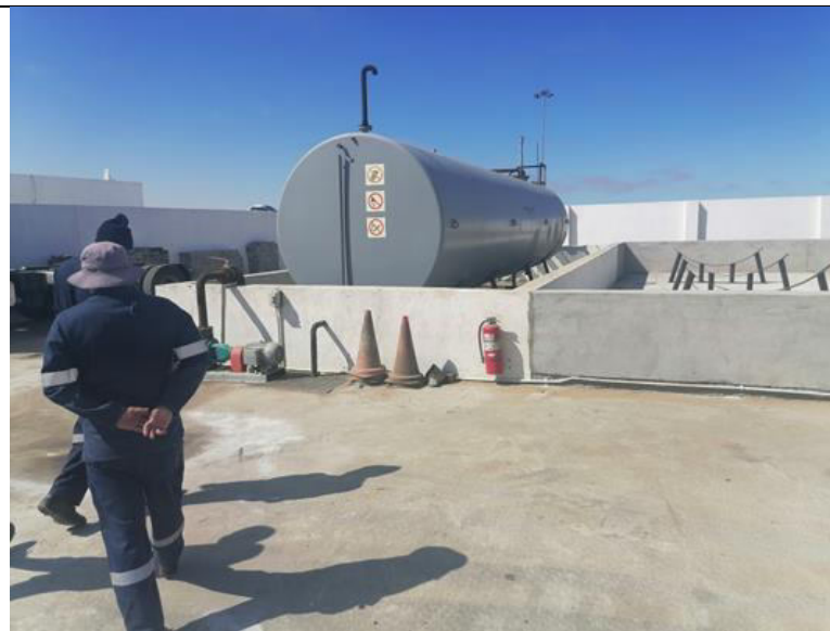
Fuel Storage tanks
