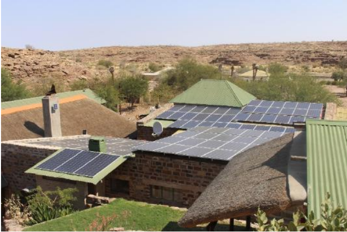
Figure 4: Solar panel on Seeheim Hotel
