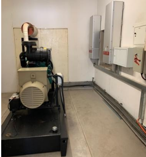
Figure 21. The generator room is sealed for noise.
