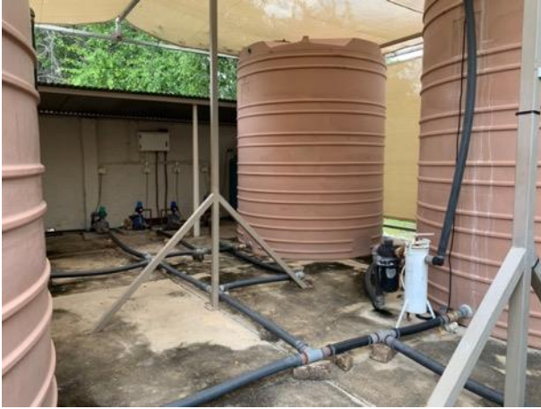
Figure 16. Water tanks on a concrete slab.
