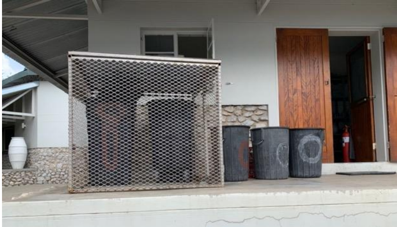
Figure 19. Rubbish bins and cage at the kitchen back door.
