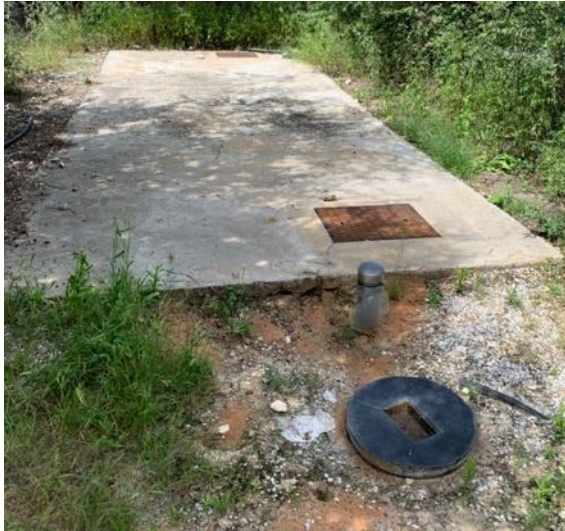
Figure 18. French drain and digester tank for the main area and guide rooms.
