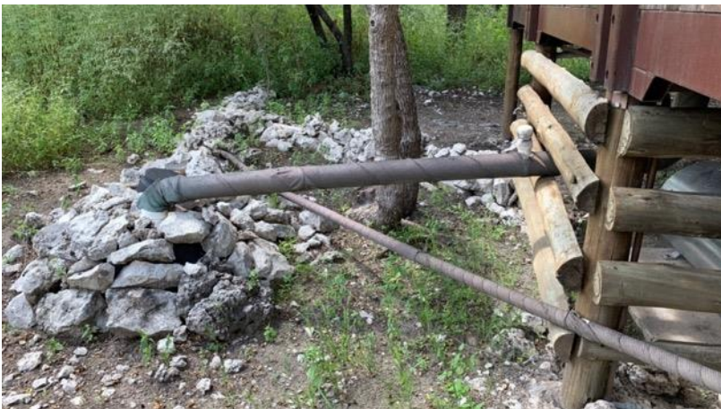
Figure 17. Pipes leading to the digester tank from a guest room.
