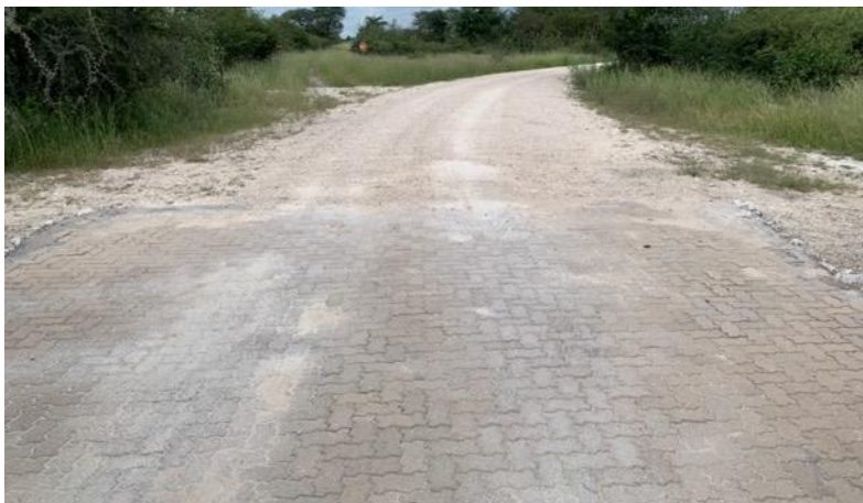
Figure 22. Road surface at the entrance gate to Outpost.
