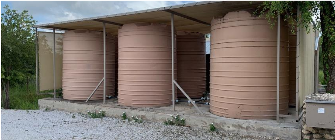
Figure 20. Six water tanks on a concrete slab.
