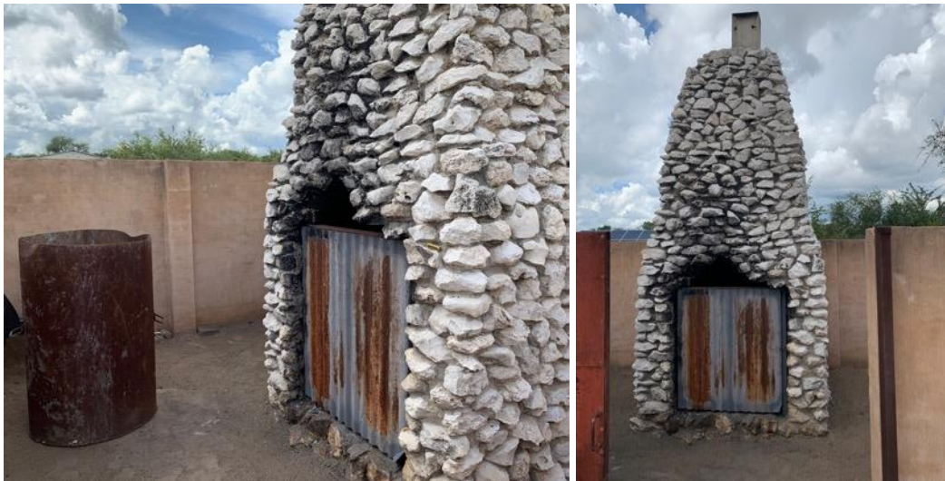
Figure 22. The incinerator inside a walled enclosure.
