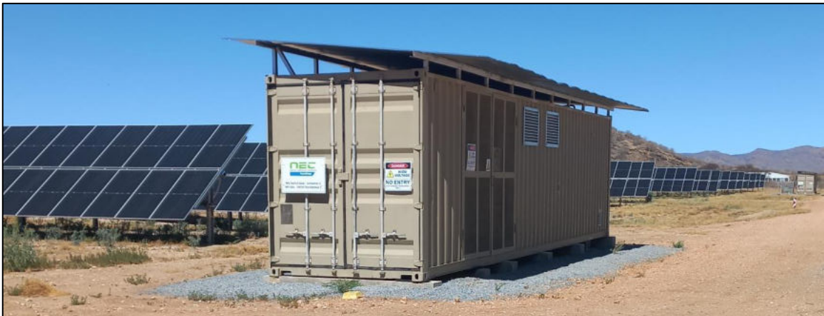
Figure 9: Power storage Transformer / Container
