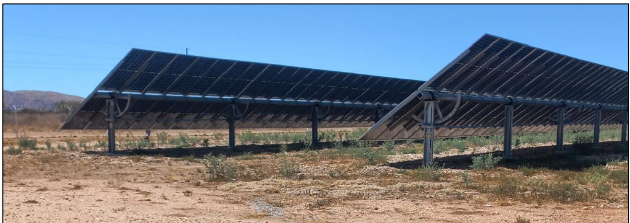
Figure 5: Solar panels on site
