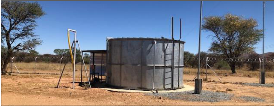
Figure 8: Water tank on site
