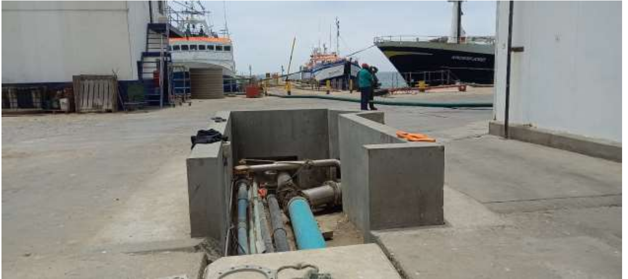
Figure 4: Pipeline Network in a concrete sleeve with the jetty terminal in the background
