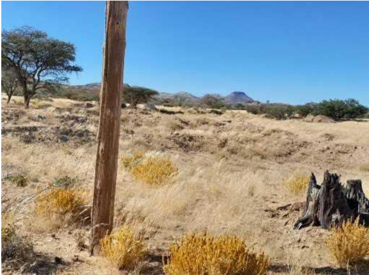
Pic 4: Uncontrolled excavation very close to electric pole (a big gully after the pole)
