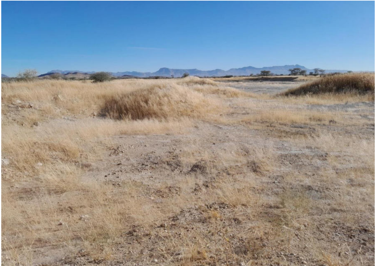
Picture 4: Further scattered heaps due to unrestrained excavation
