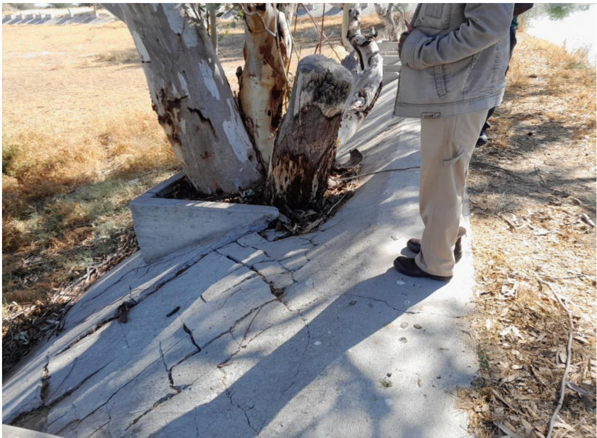
Pic 8: Integrity of pond compromise due to growing trees
