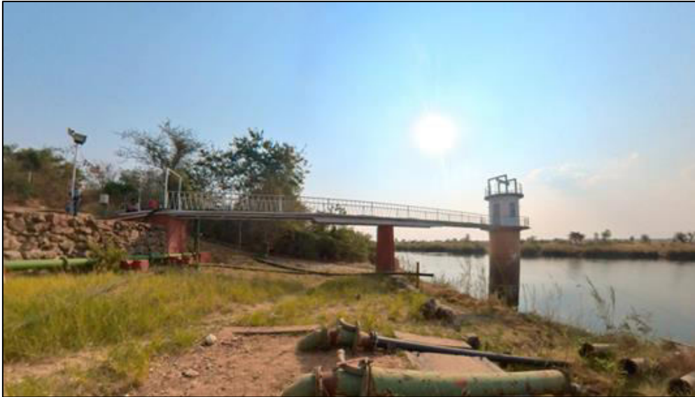
Figure 2-5: Rundu Abstraction Tower
