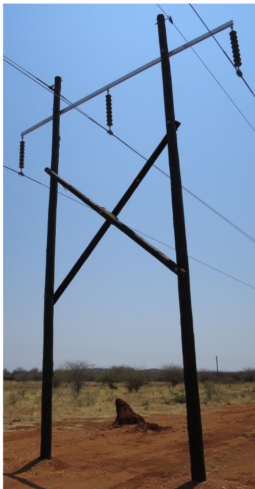
Plate 2.1: Example of the 66kV wooden structure with wooden crossarm (Source: Transmission Consulting Services (TCS), 2020).
