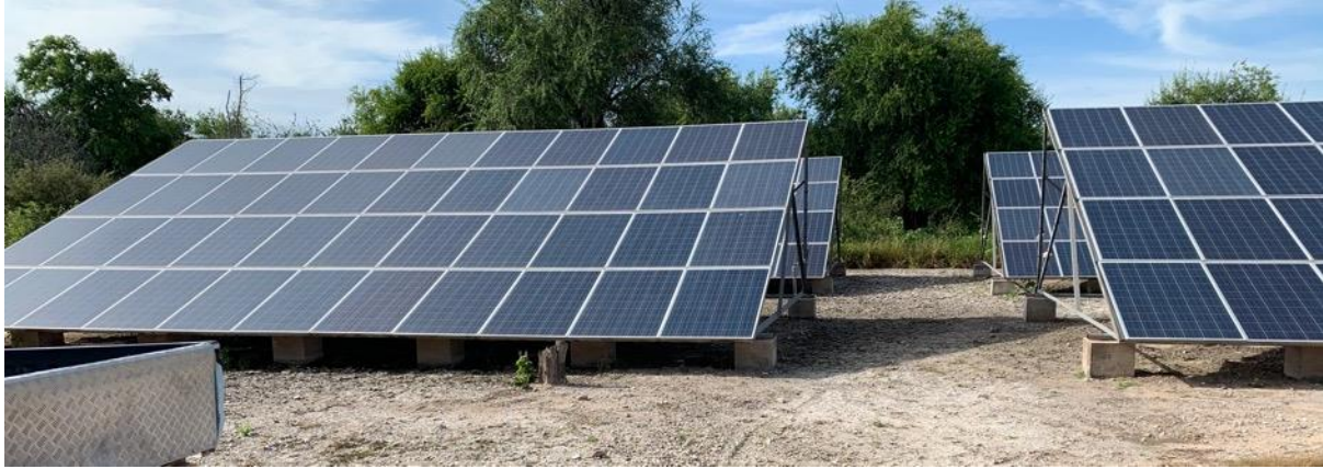
Figure 45. Four solar panels feed into the grid.
