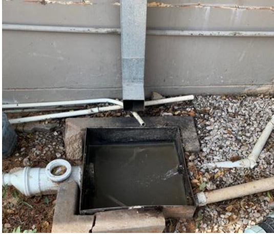
Figure 39. Fat trap at the kitchen drain outlet.
