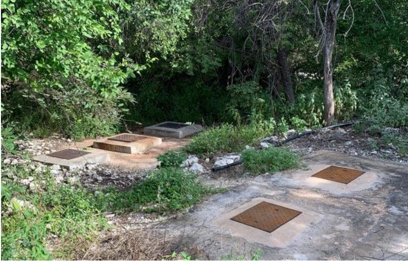
Figure 36. The staff village sewage drains into two systems.
