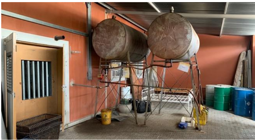
Figure 19. Fuel tanks and the door to the generator room.
