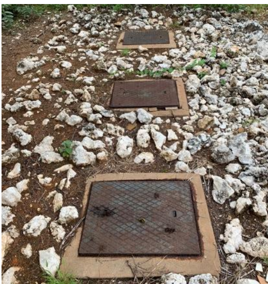
Figure 38. One of eight French drains servicing the guest rooms.
