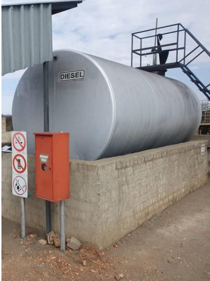
Figure 1: Above Ground Engen 23 000 L tank
