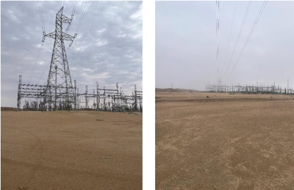
Figure 4: OHL Pylons connecting to Lithops Sub Station
