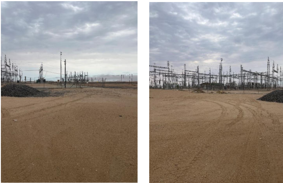
Figure 5: Existing Lithops Substation and access road to be used for OHL ROW
