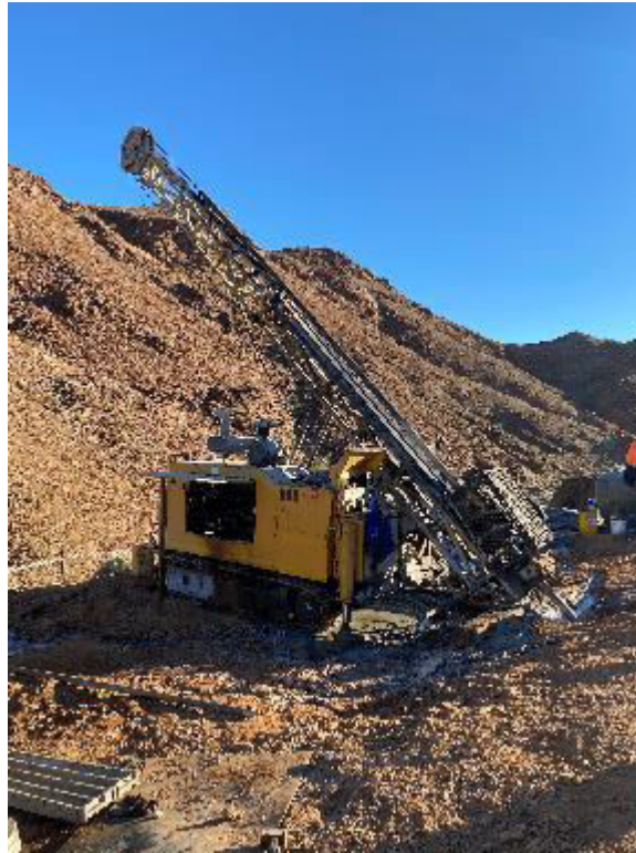
Figure 5: Example of a drill rig used on site (established in previous years at the Haib site)
