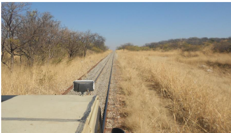
Figure 2. Vegetation that has grown too close to the railway line
