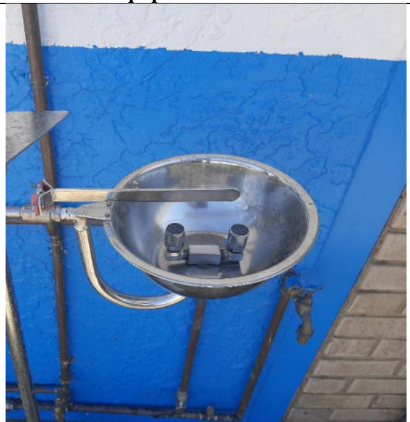
Photo 4-6 Emergency eyewash station
