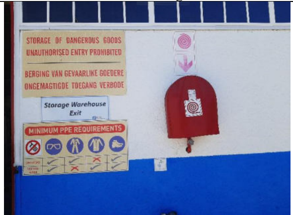
Photo 4-4 Safety signage and firefighting equipment
