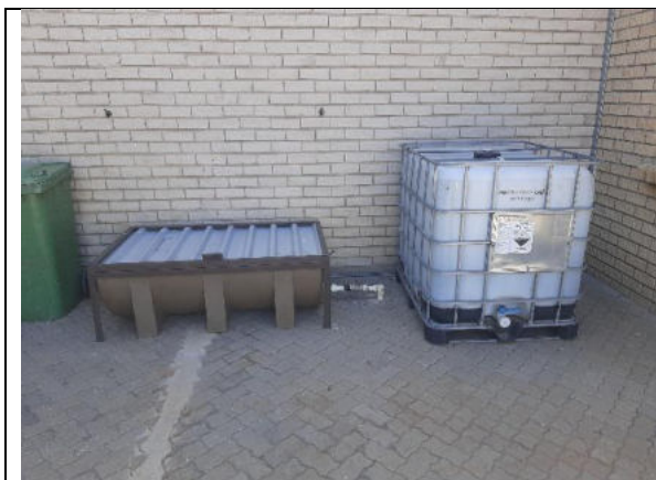
Photo 4-7 Emergency water bath with water storage
