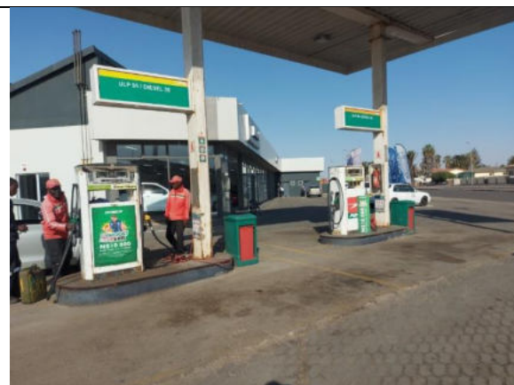
Photo 4-2 Pump islands under canopy
