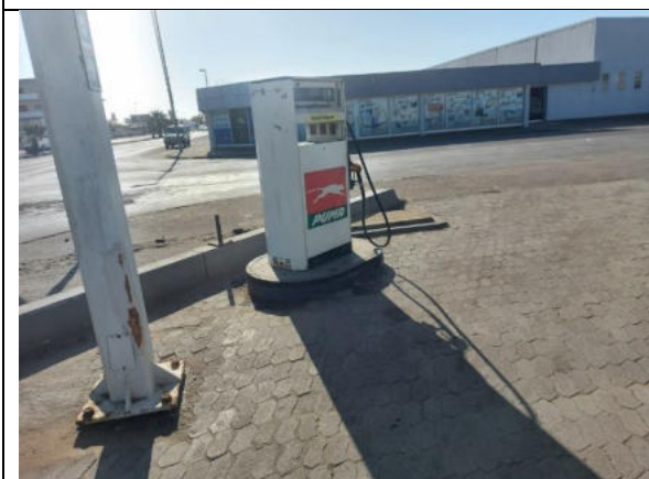
Photo 4-3 Pump island – diesel only
