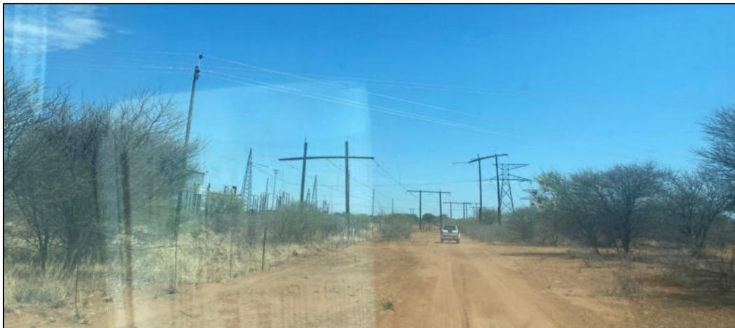
Image 1-8: Existing overhead powerlines
