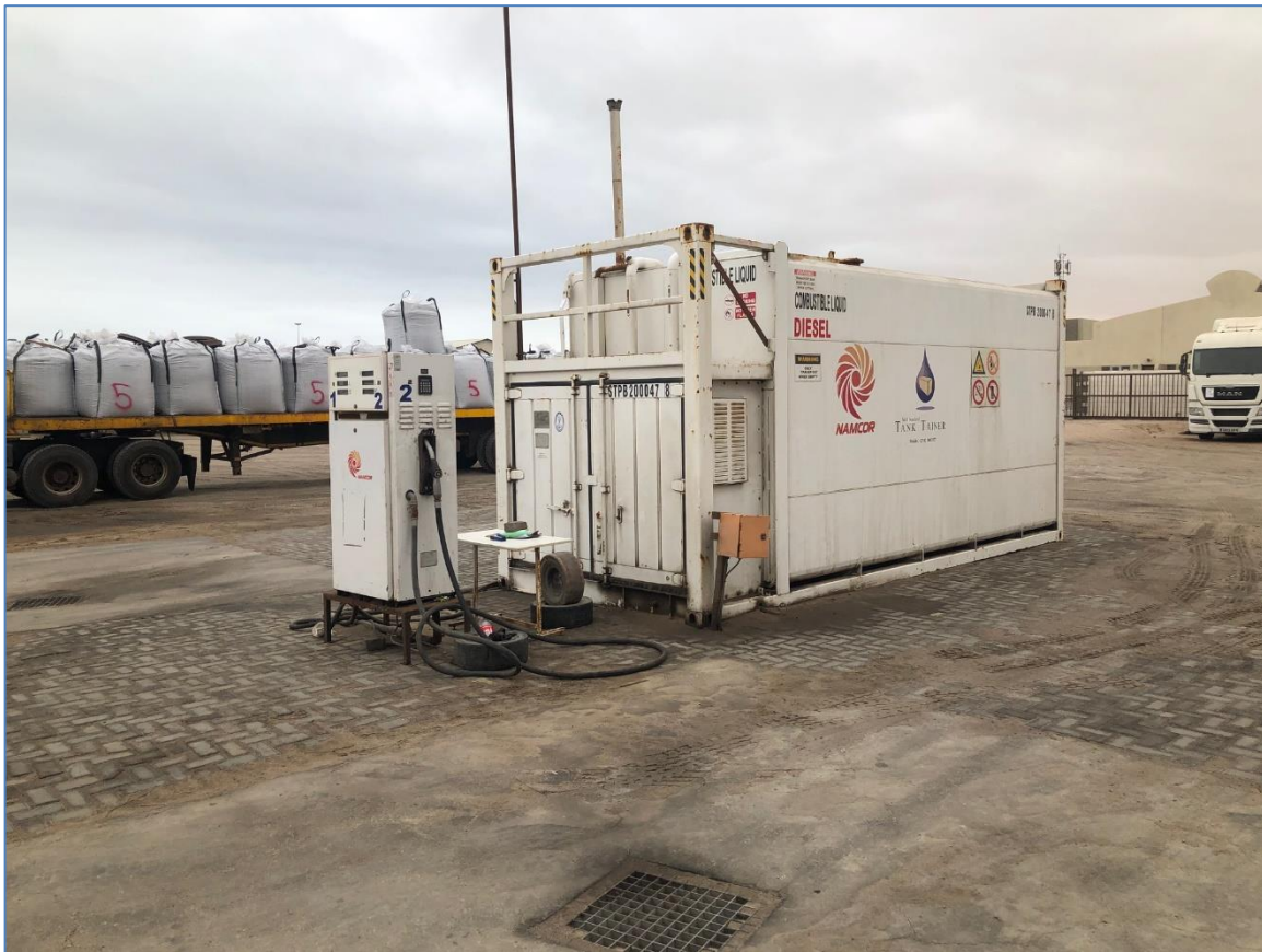
Figure 9: Existing diesel tank and pump
