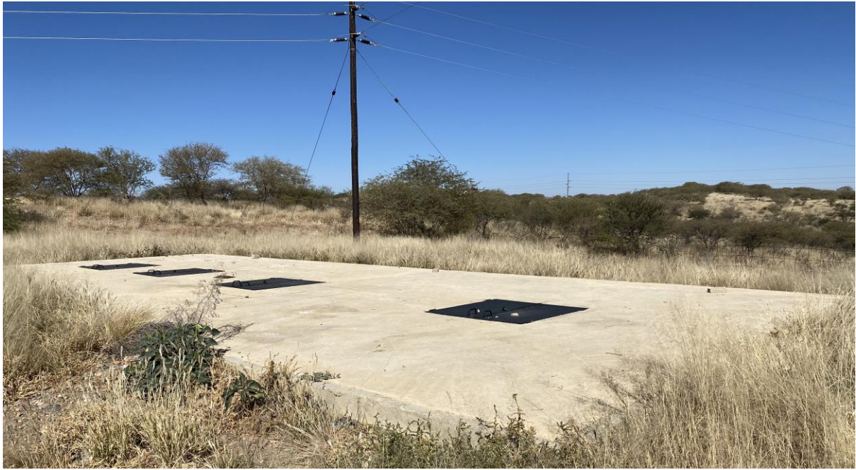
Figure 1.3: Onsite Septic Tank for Wastewater management
