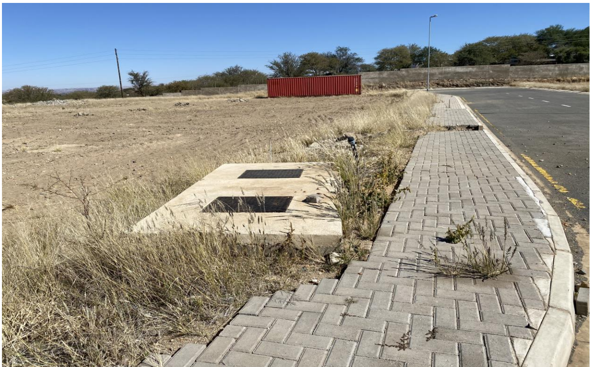
Figure 2.4: Series of Wastewater management septic tanks
