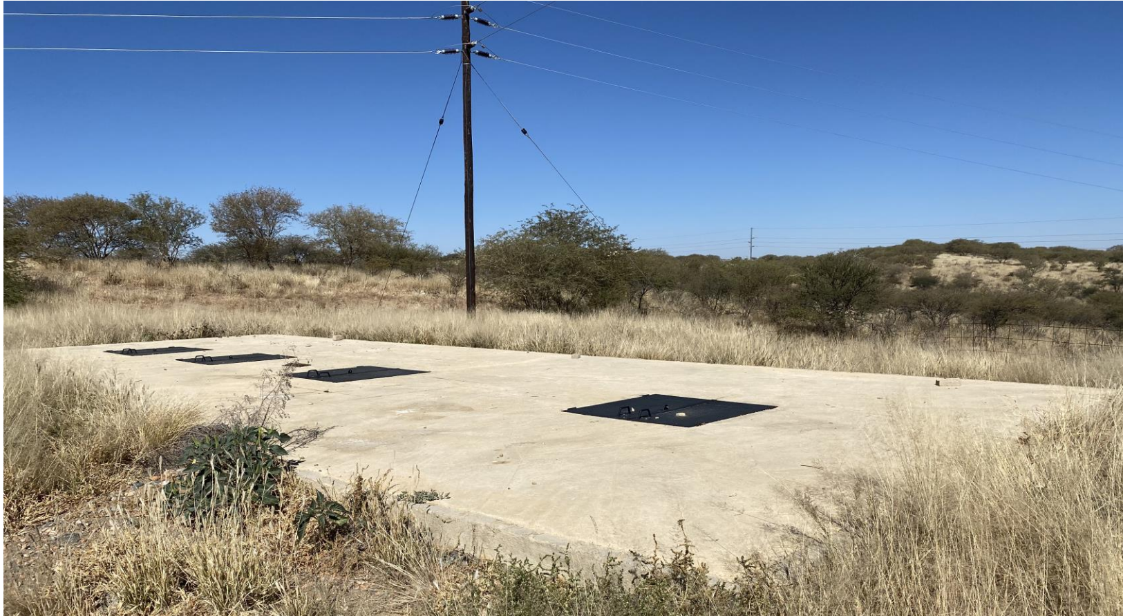
Figure 2-3: Onsite Septic Tank for Wastewater management
