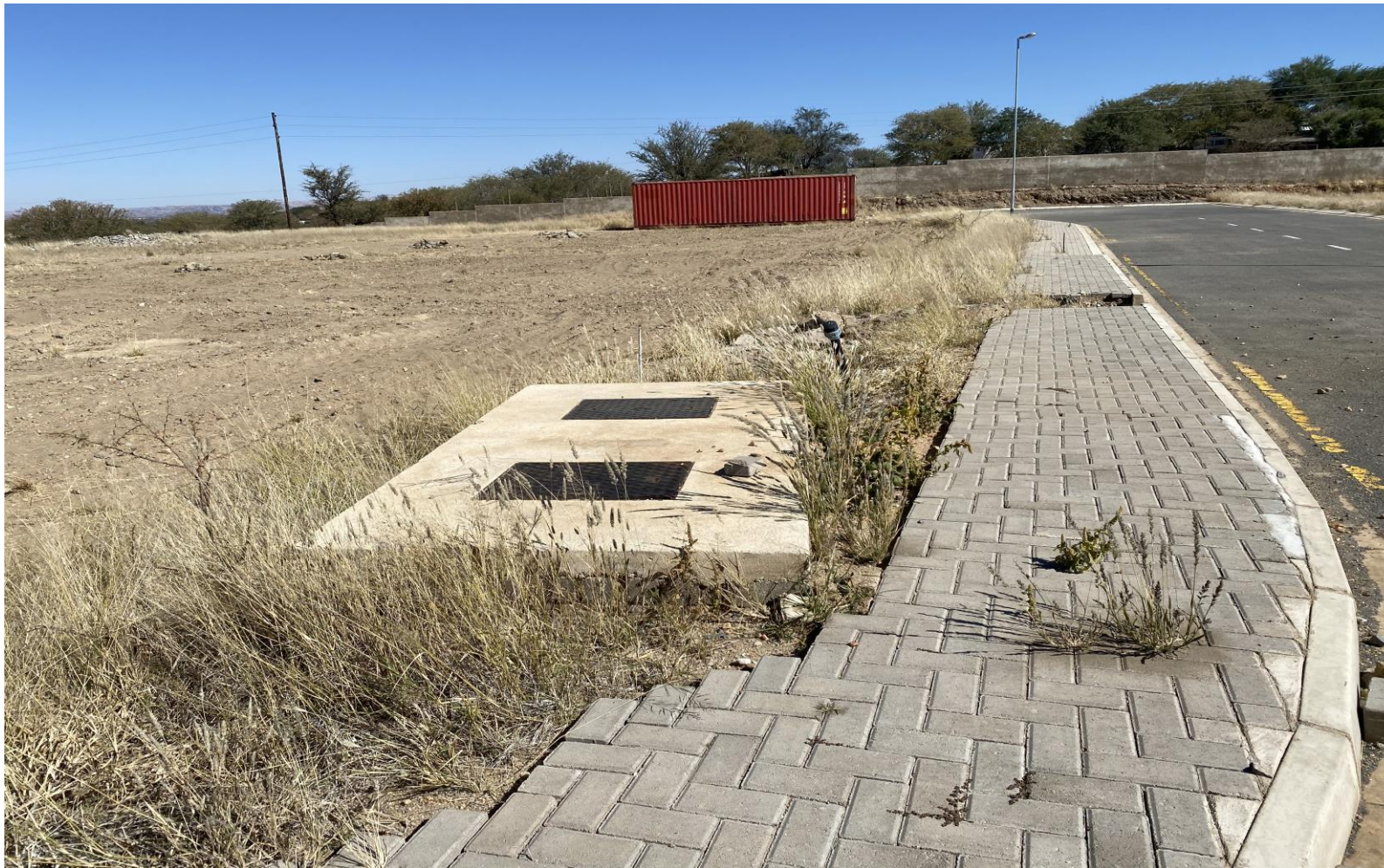
Figure 2-4: Series of Wastewater management septic tanks
