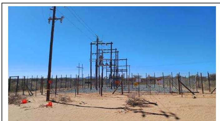
Photo 4.3.2-1 – View of existing Sungate Substation
