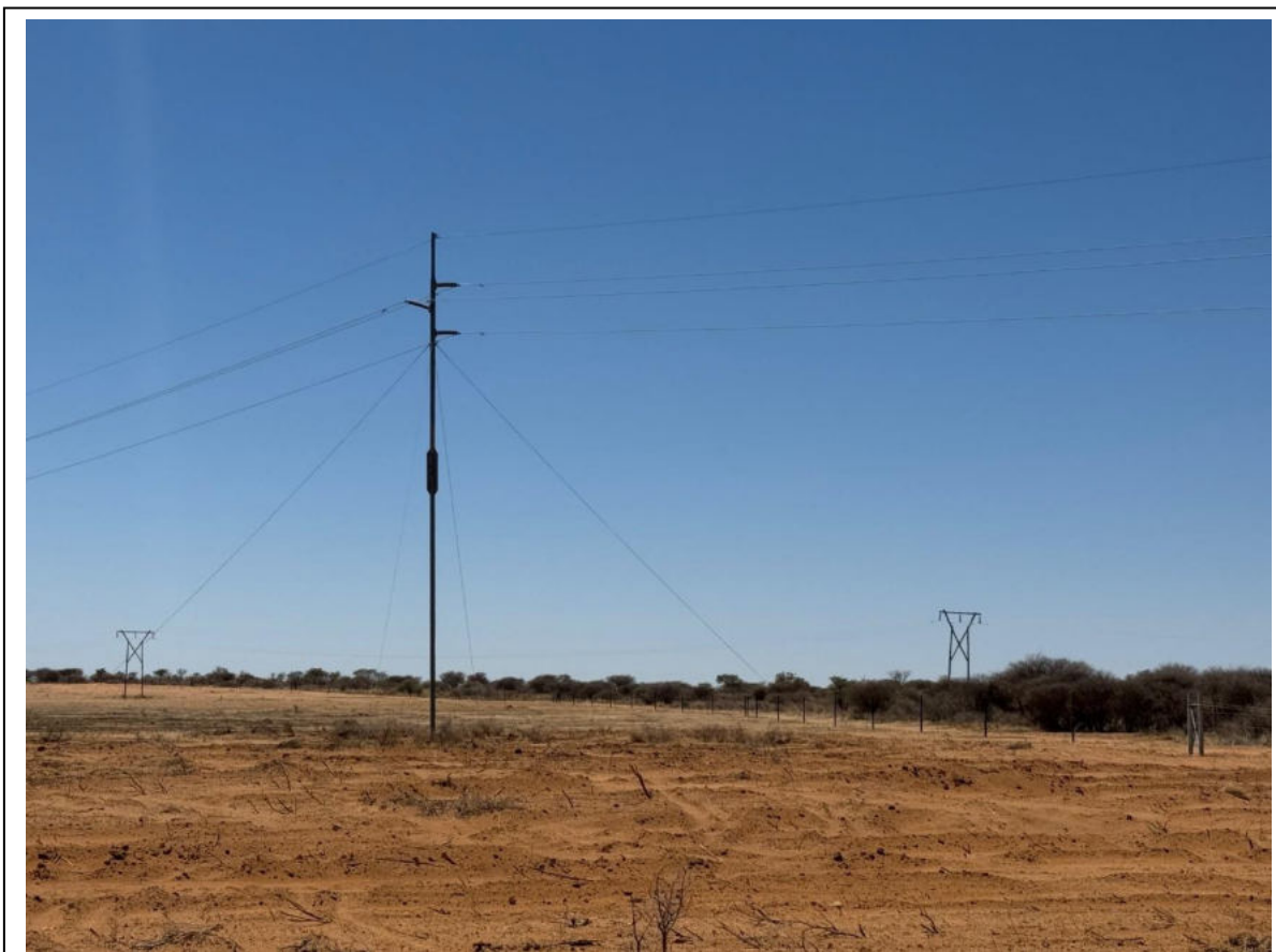
Photo 1 – View of existing 132kV OHTL (front) and existing 66kV OHTL (back).
