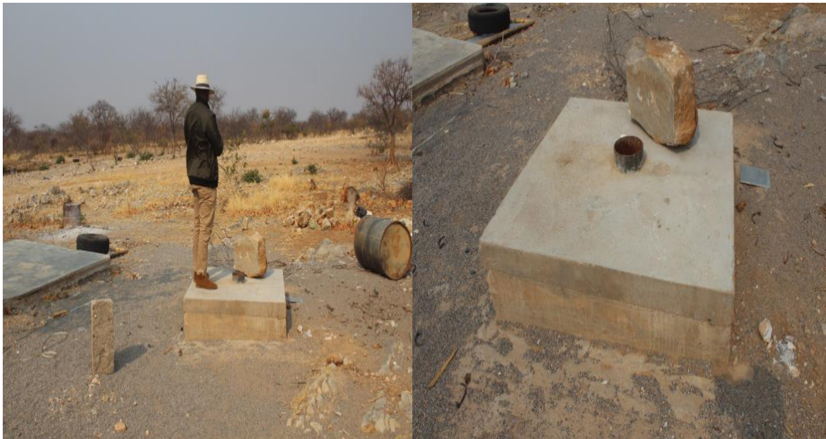
Figure 2: The existing borehole on Portion A at Farm Voluteer 106, that will be rehabilitated and retrofitted.
