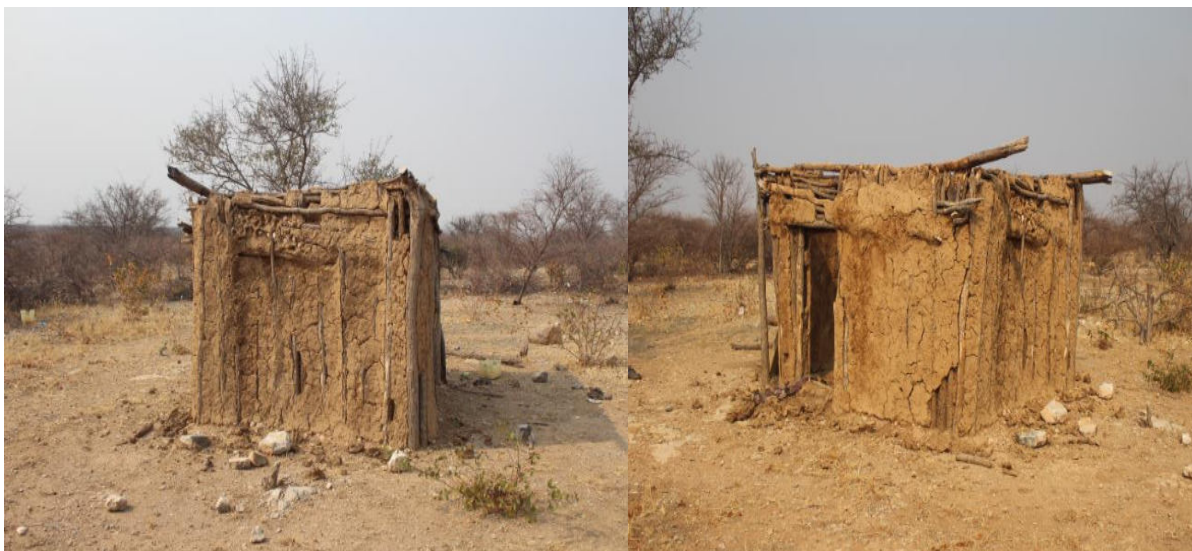
Figure 3: The existing structure on Portion A at Farm Voluteer 106, that will be demolished and upgraded to staff houses.
