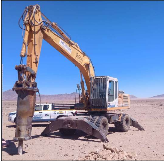
FIGURE 10: EXAMPLE OF HOW THE HOLES FOR THE UPRIGHTS WILL BE CREATED BY HAMMERING HOLES WITH A MODIFIED EXCAVATOR / JACK HAMMER
