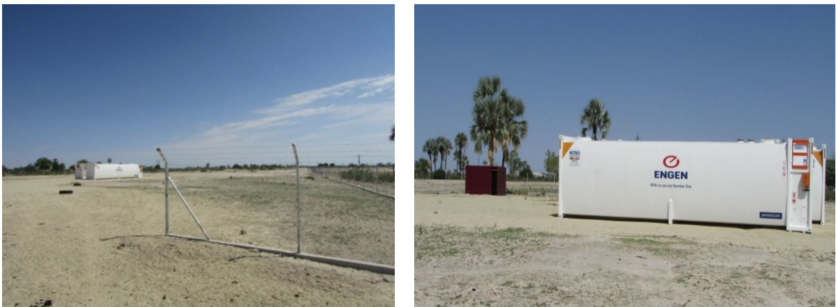
Figure 1: The site view with the two mobile fuel units
