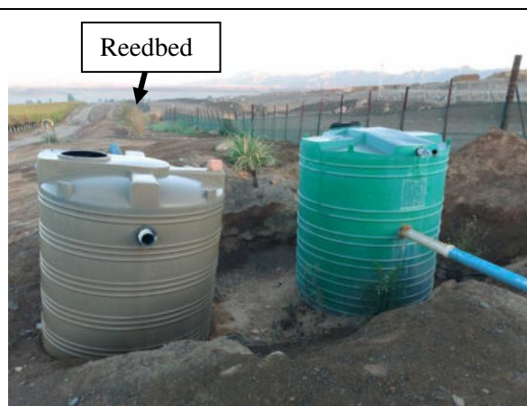
Photo 5-10 Chlorination tank (green) and reedbed (brown tank now removed)
