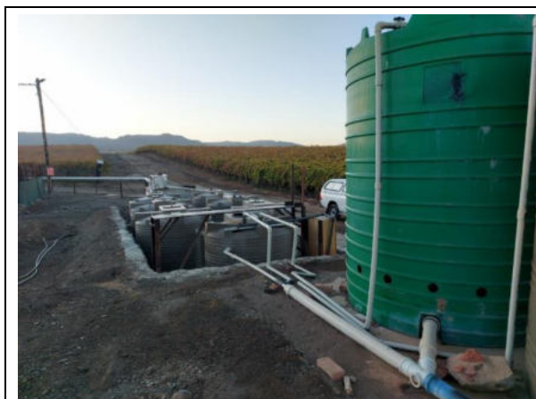
Photo 5-5 Wastewater treatment plant
