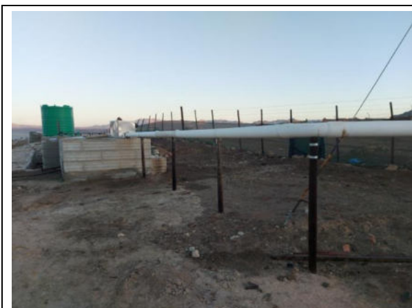
Photo 5-7 Sewerage main (waste water pipeline) leading to sewage treatment system
