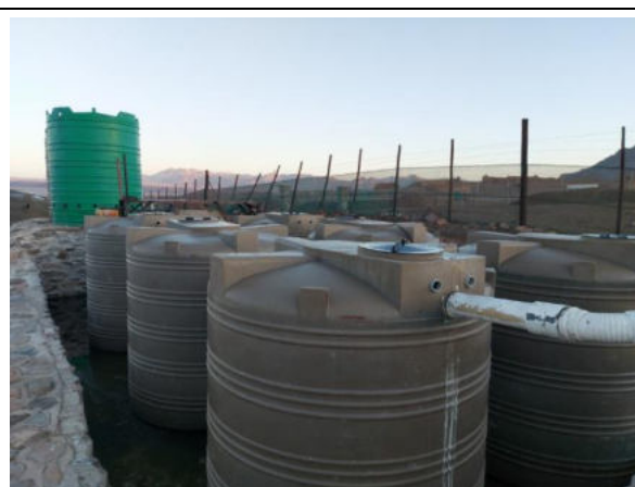
Photo 5-8 Septic tanks (brown) and trickling filter tank (green)
