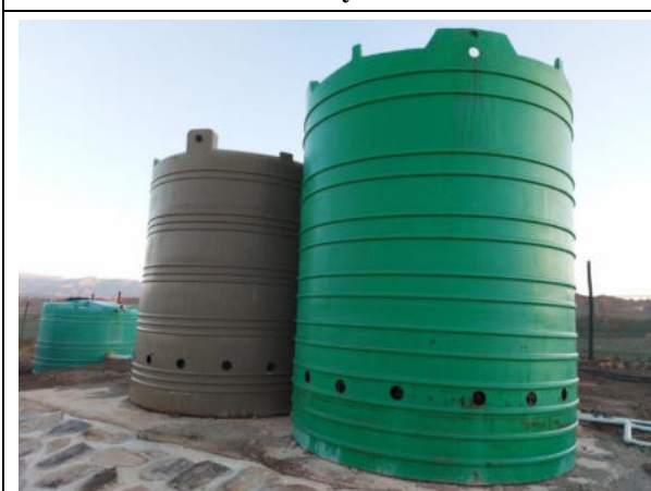
Photo 5-9 Trickling filter tanks
