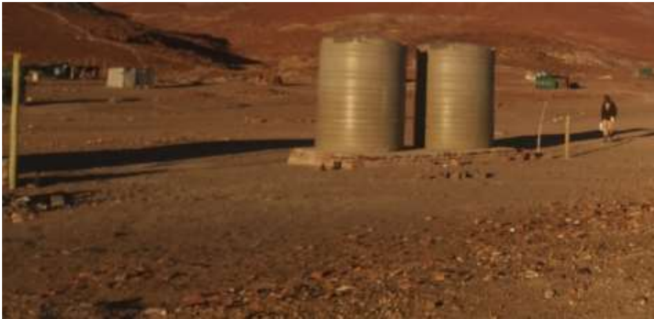
Figure 9: Water storage tanks
