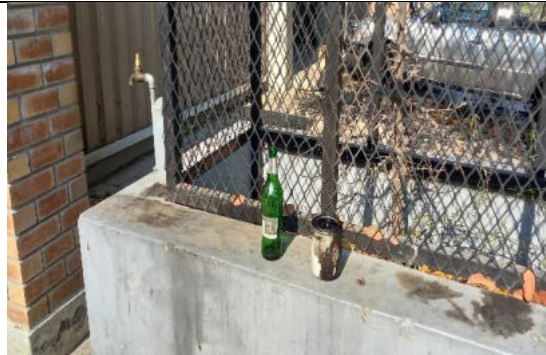
Figure 20: Tap Water & Oil Stained Walls
