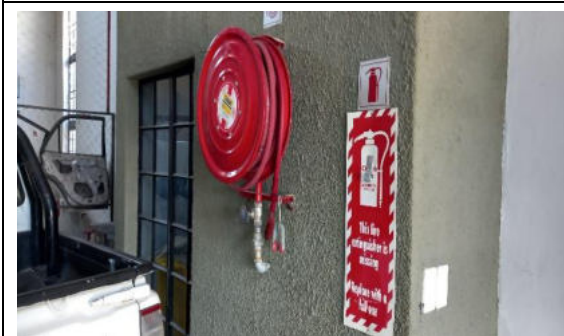
Figure 19: Fire Fighting Equipment
