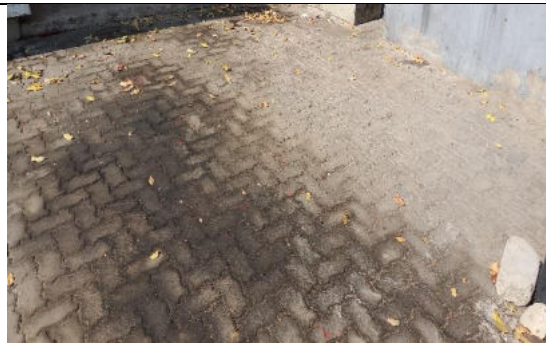
Figure 18: Oil Stained Floors
