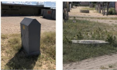
Figure 3: On Site Utility Services
