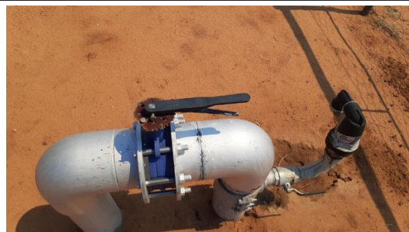
Photo 4-13. Borehole cut-off valve on Anaboom No. 400 (Portion 1)
