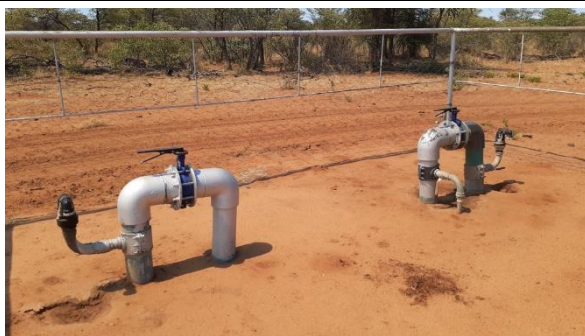
Photo 4-12. Borehole cut-off valves next to installation at chemical mixing tank on Anaboom No. 400 (Portion 1)
