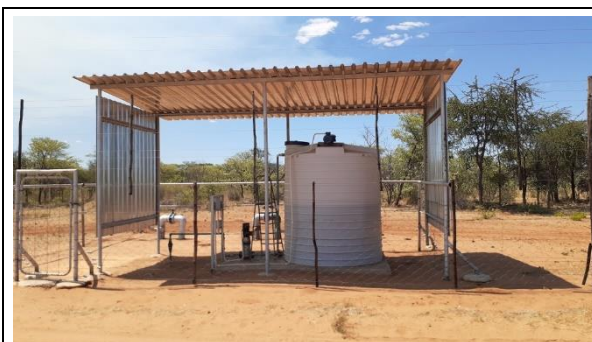
Photo 4-3. Fertilizer mixing tank on Portion 1 of Anaboom No. 400
