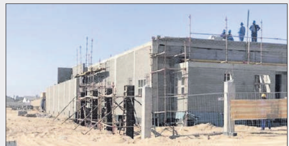
The Paratus landing station will host the Equiano undersea cable system transmission equipment.
