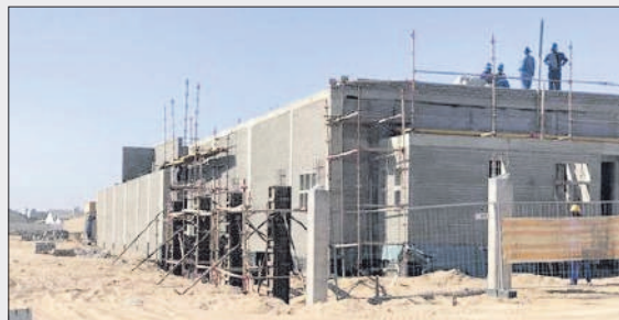
The Paratus landing station will host the Equiano undersea cable system transmission equipment. PHOTO CONTRIBUTED
