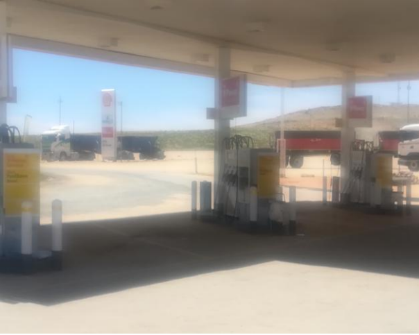
Photo 1. Existing dispensing points, forecourt and canopy
