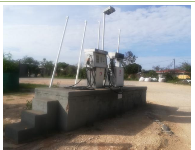
Photo 2. Existing dispensing points- Unoperational
