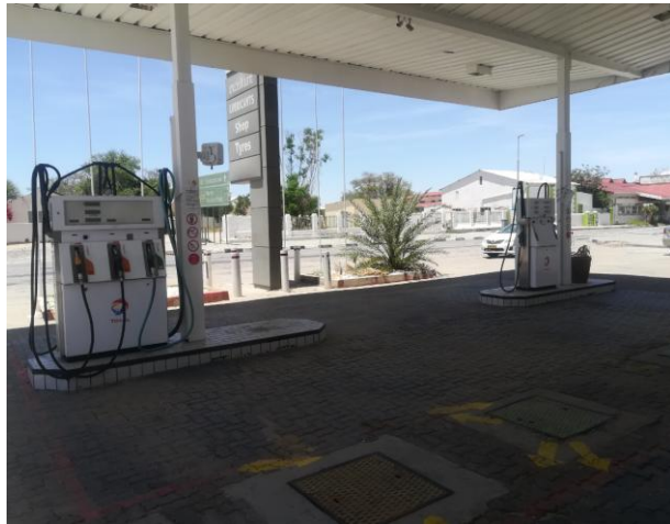
Photo 2. Existing dispensing pumps with islands
