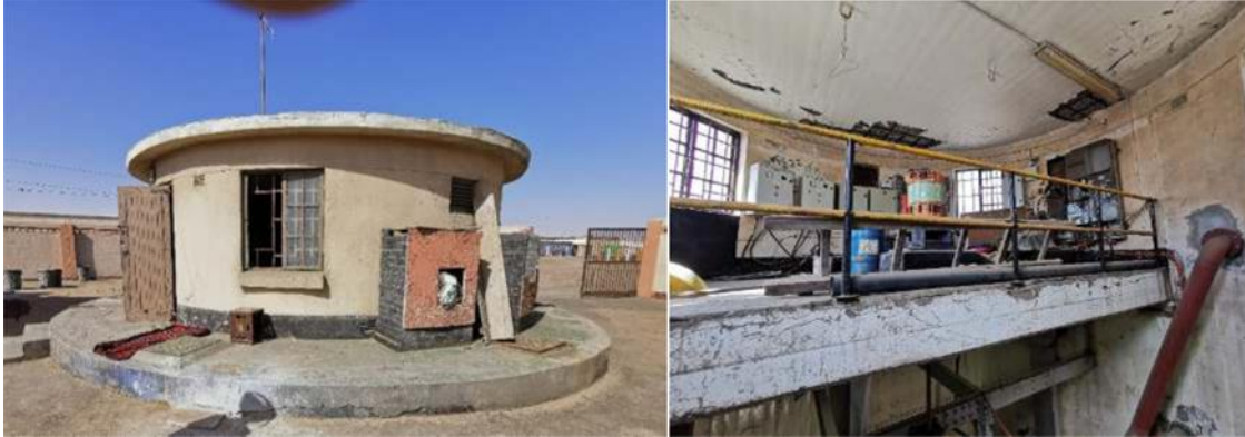
Figure 10.3: Civil/structural condition of Kuisebmond existing pump station
